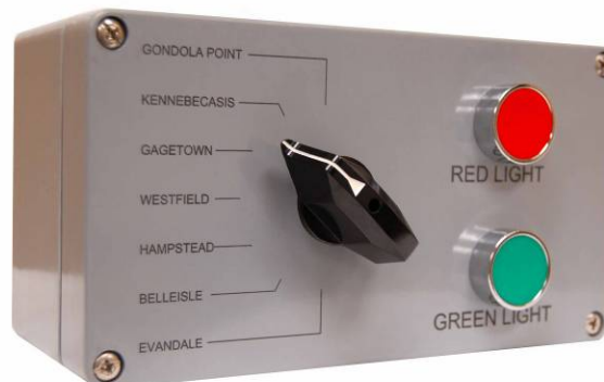
Figure 1: Ferry-side Controller Front Panel
