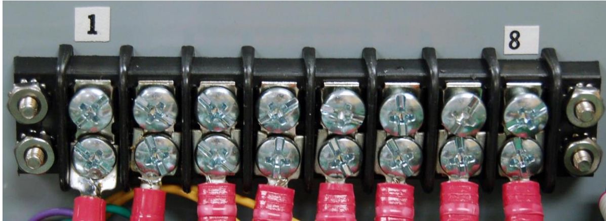
Figure 1: Image of Terminal Strip inside Industrial Controller
